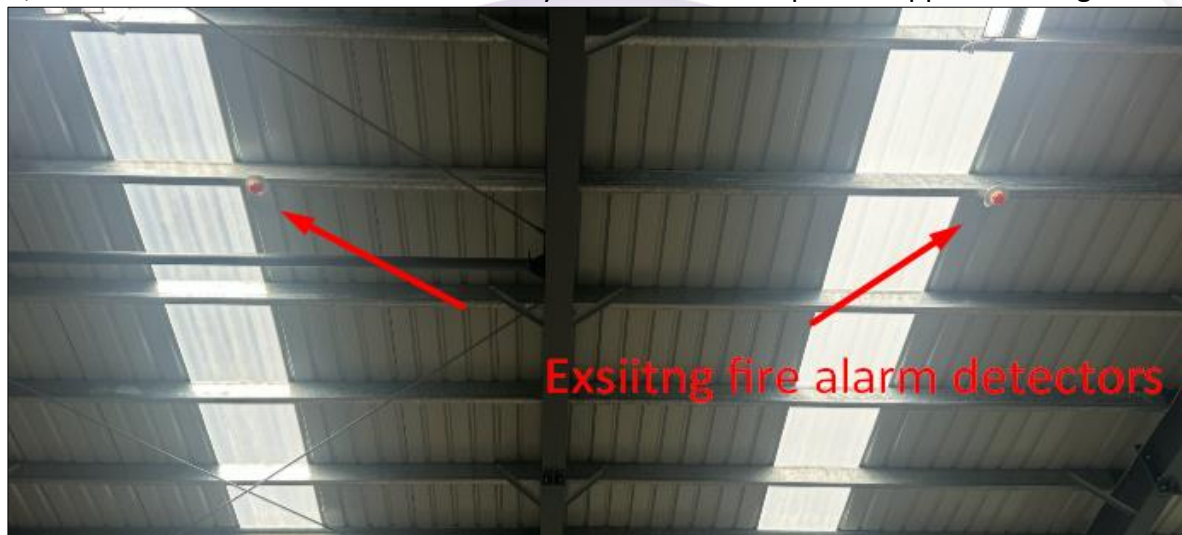
Picture 1. Existing fire alarm detectors (G-Store -1)
